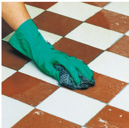
Use a suitable cleaning agent to remove residues - which could impair adhesion - from the substrate.
